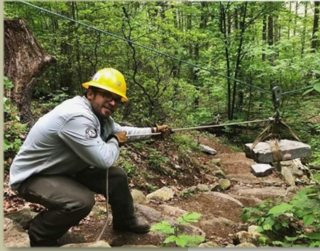
A photo of Eli using a griphoist high line to build a rock staircase in Leominster, MA.
